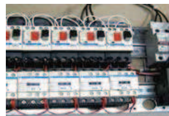
The electrical system is easy to service. The electric cabinet is located at a comfortable working height and all the components are clearly labelled. The system is carefully designed with a logical layout.
